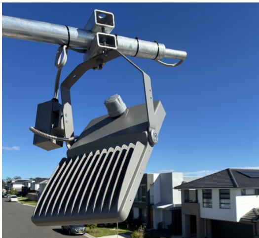
This image shows the floodlight and connection box mounted incorrectly
